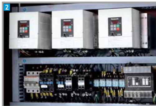
Electric Control Unit
